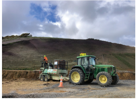
Hydrosoil is hydraulically applied as a slurry from truck mounted hydros seeding units.
